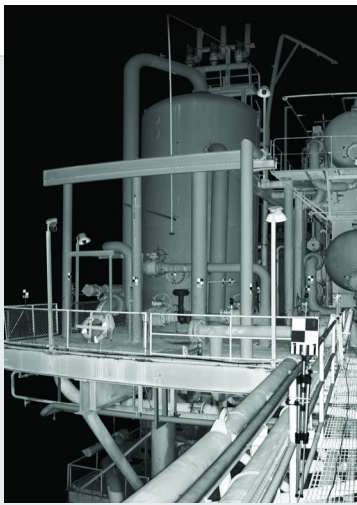
Intensity image taken from a laser scan of an offshore production platform.
