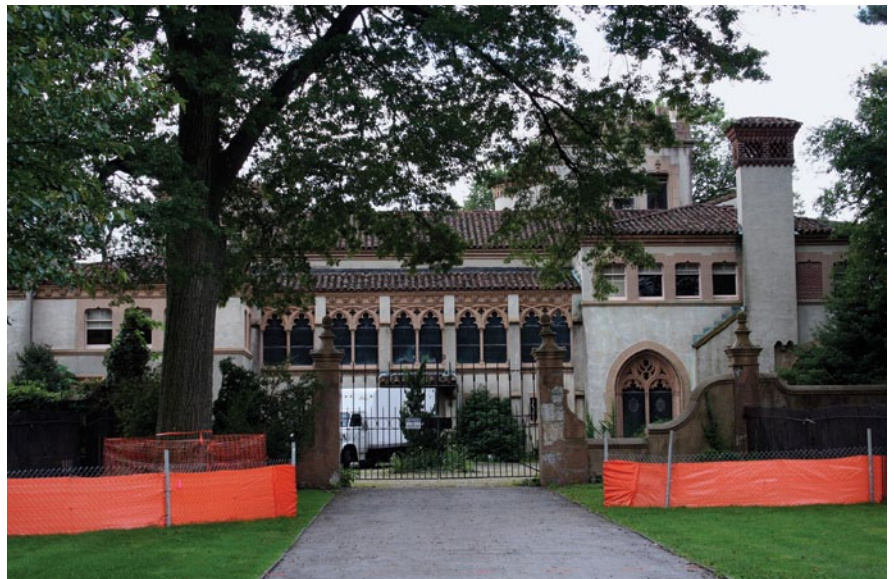
Sept. 10, 2009: The silt fence is up, trucks are on site presumably to cart away some of the interior features during gutting, but in this “pre-demolition” scene La Ronda still looks intact from the outside.
